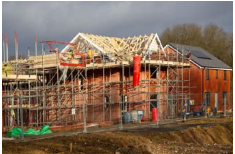
Persimmon housing estate Suffolk, UK trial schemes for net zero homes, and engagement with smaller suppliers on the transition.
